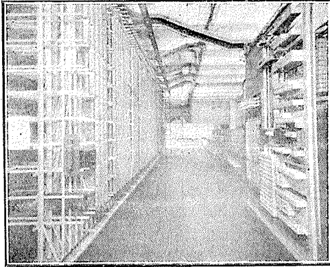
MAIN DISTRIBUTION FRAME AND TEST DESK.
