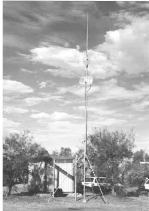
Mt. Barry radio linked telephone S.A.
