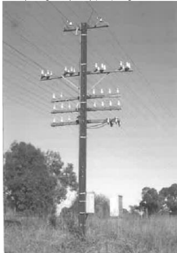
Railway telephone and control lines at Boralla, Victoria (2002)
