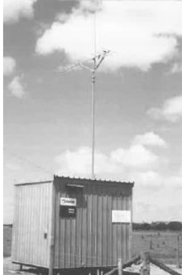
Rural Automatic Telephone Exchange with radio telephone link to some subscribers, South West W.A.
