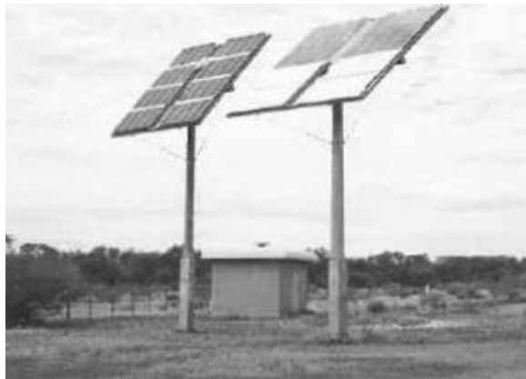
Solar powered fibre optic repeater besides the Stuart Highway northern Australia.
