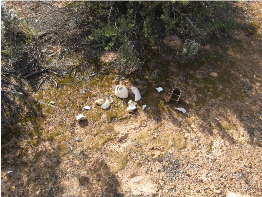
E W telegraph line where it crosses Eyre Highway Broken insulators
