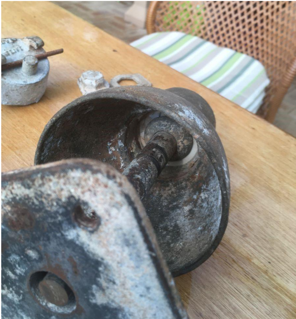
Metal cap glued on broken insulator top
