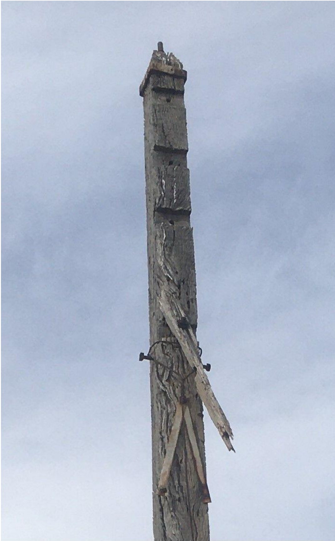
Pole 1 Top section
