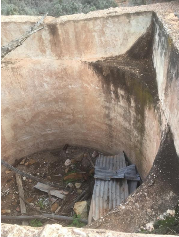
2021. Cook's house. Underground water tank.
